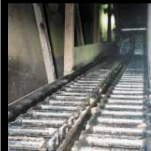
Chip Reclaim Conveyor
