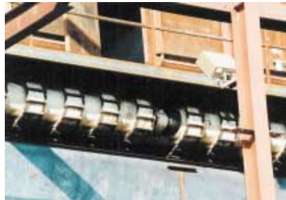
Live Bottom Bin, Waferboard Plant
